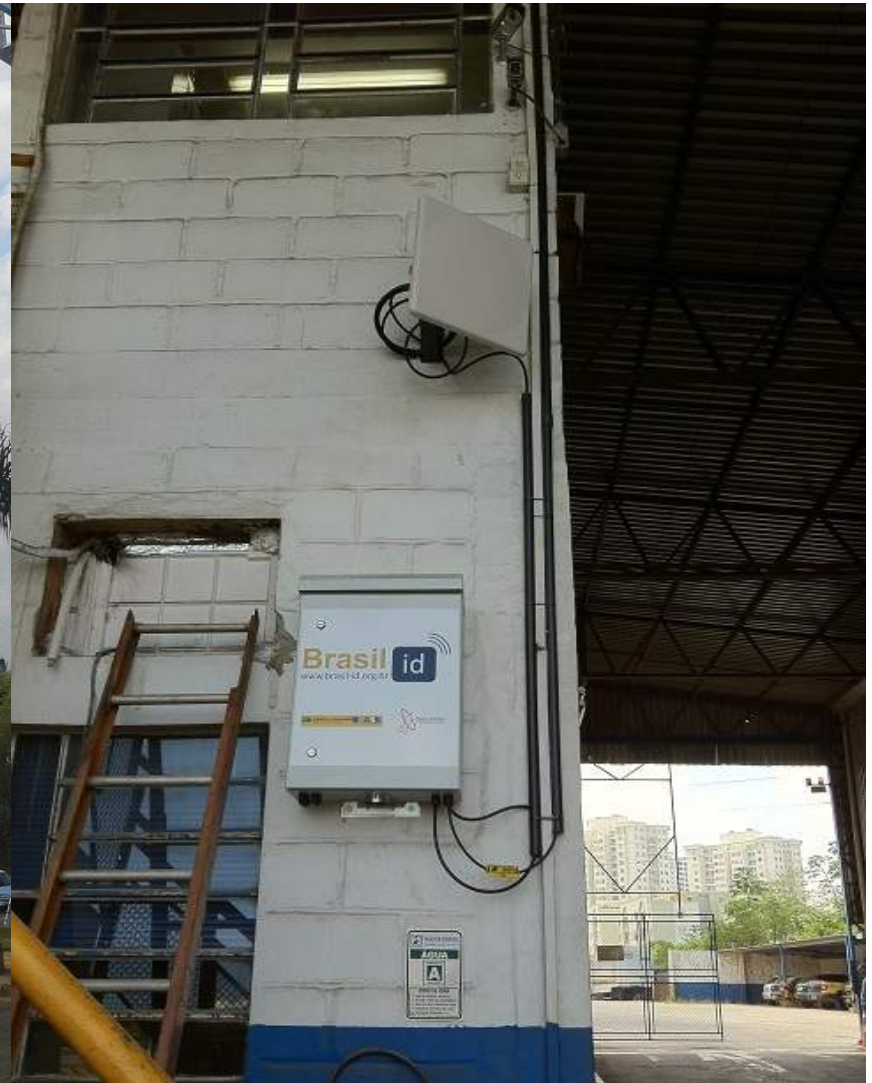
VBL's Road-Side Equip being installed at a company's facility
